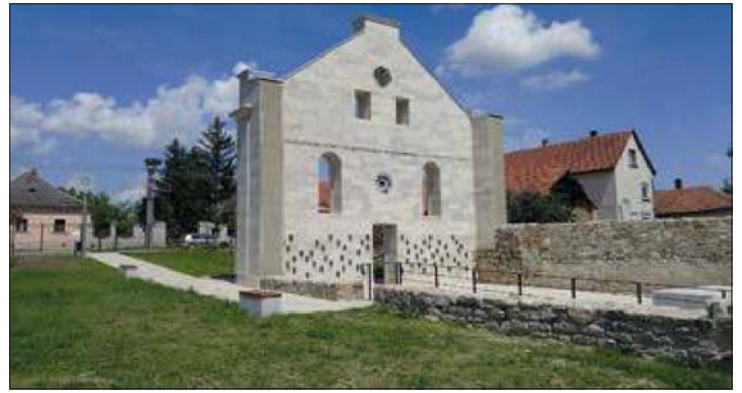
Footprint of the shul interior area, with a view of the newly constructed entrance wall
